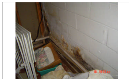
Mold growth in North corner interior where outside ditch is located
