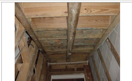
Mold growth on wood stairwell due to excessive humidity in basement
