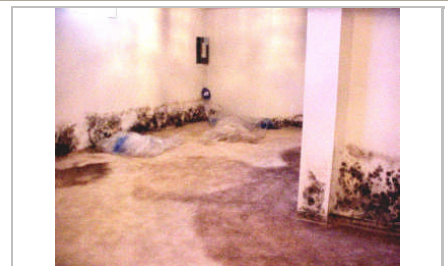
Fix ditch or else this will happen!
